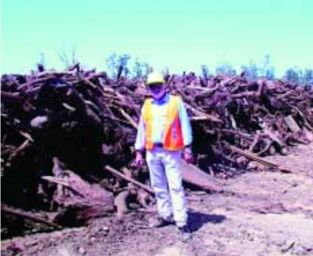
Alcoa mine site clearing residue heap, ready for processing to alternative uses such as mulch or charcoal.
