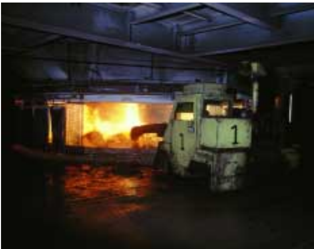
27 MVA Submerged Arc Silicon Furnace.
